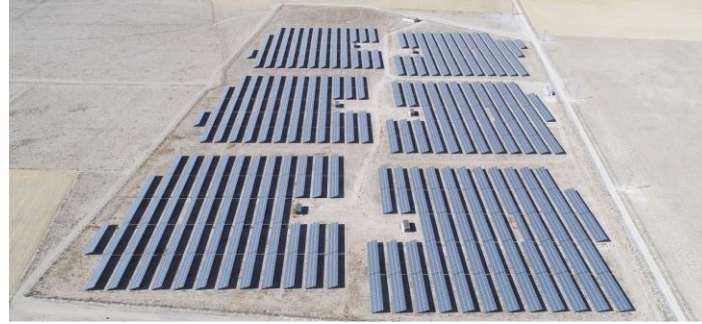
UZUNKUYU SOLAR POWER PLANT Established DC Power: 10.361,50 kWp
