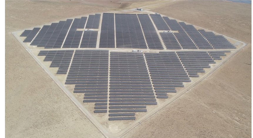
PSI ENGI207 SOLAR POWER PLANT Established DC Power: 12.969,18 kWp
